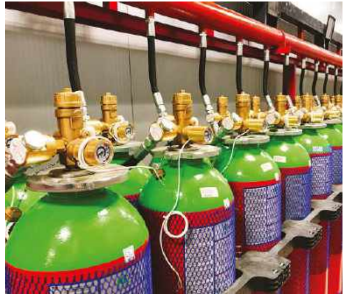
Fire suppression systems
